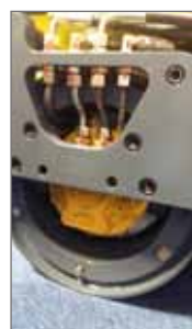
Two hydraulic Poclair pumps
